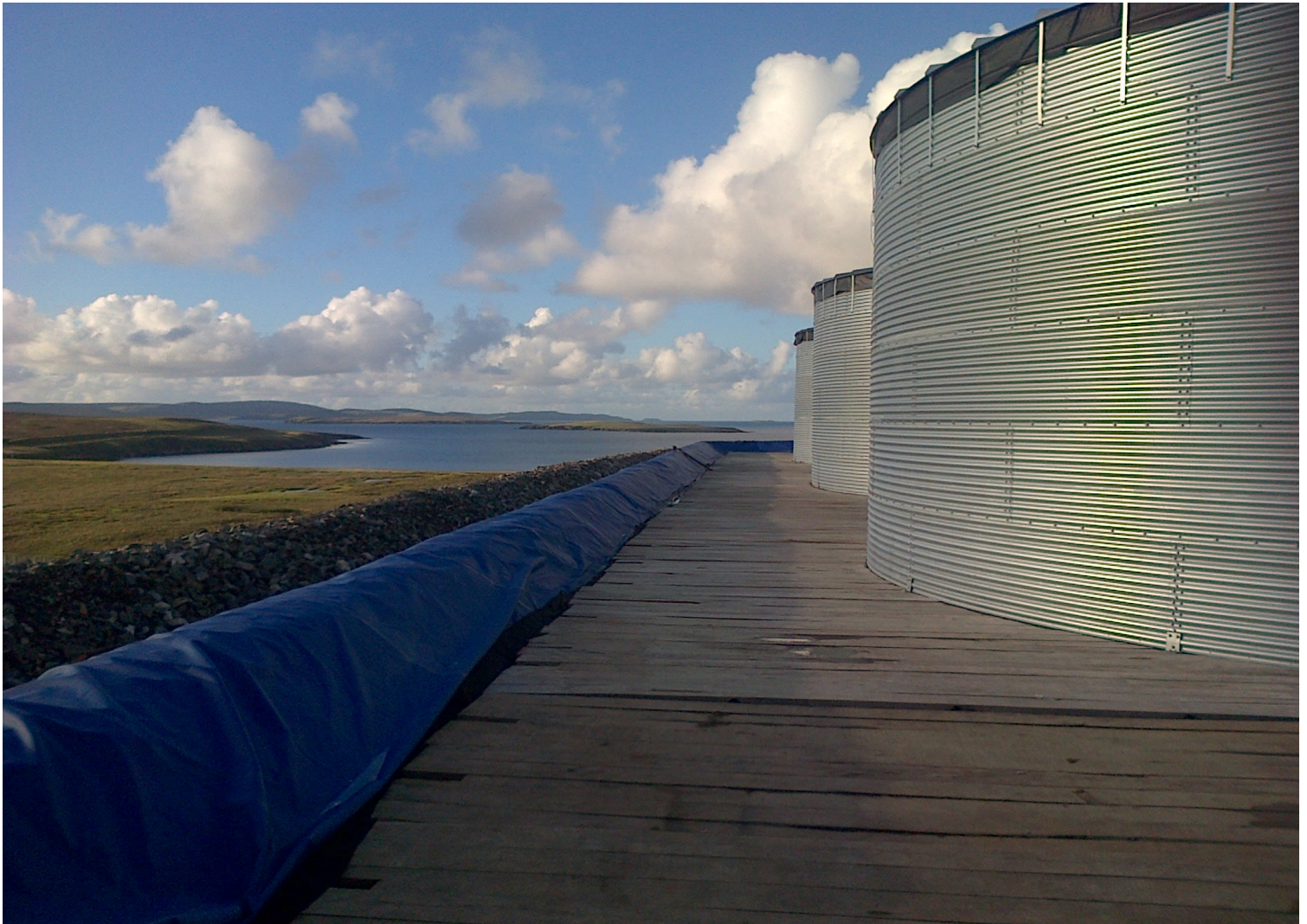
Deployed tanks with secondary containment (blue PVC) bund lining visible on the left
