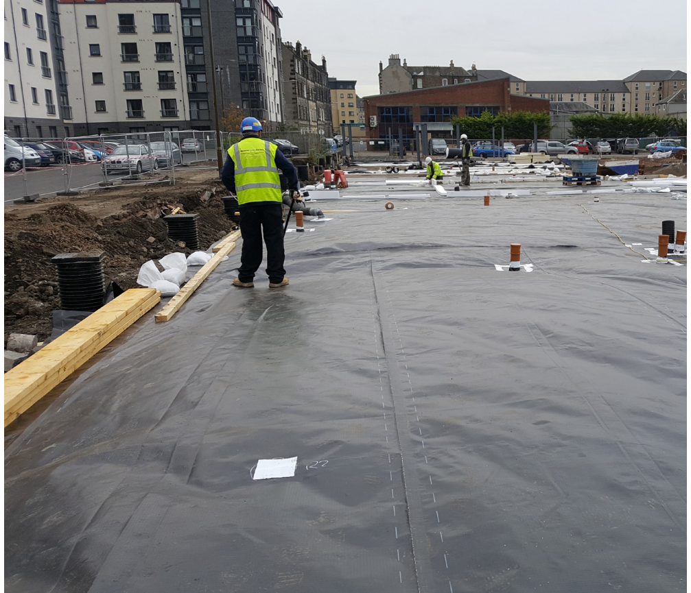
Above left: Independent air lance integrity testing to installed Landflex ZR60 gas membrane Above right: Independent tracer gas testing of first block in accordance with local authority requirements
