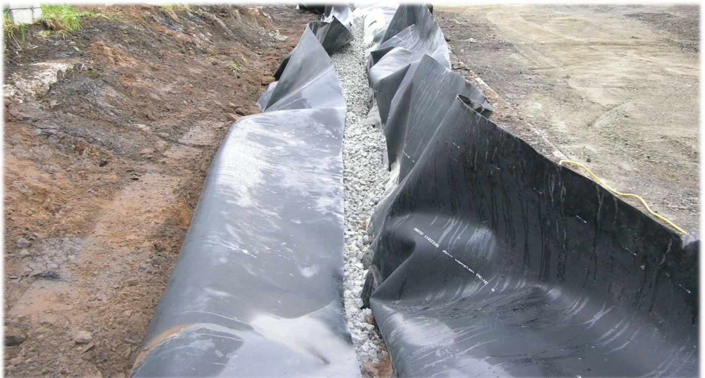
Filter Trench Linings—Stone Filled or Crate Systems Supply & Install or Supply Only
