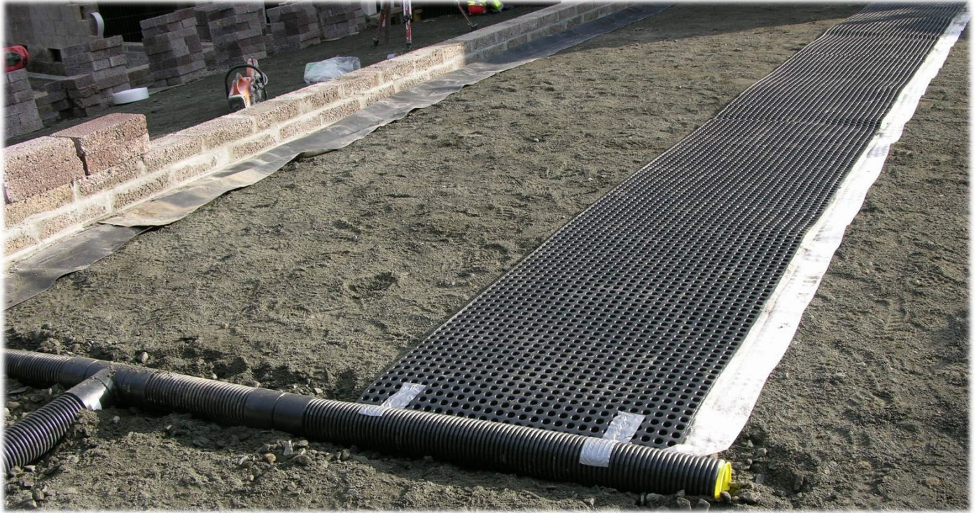
Gas Venting Systems—Design, Supply & Installation
